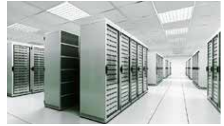
DC-powered data center of green.ch in Lupfig, (Source: Securiton)
